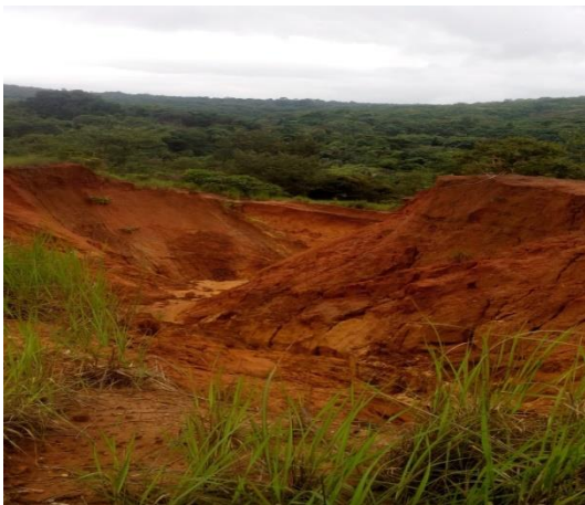
Plate 3; Gully site at Akpo (Otaalu)
