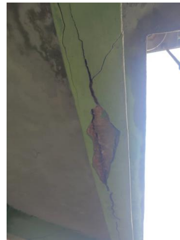
Fig. 5 Crack along the beam
