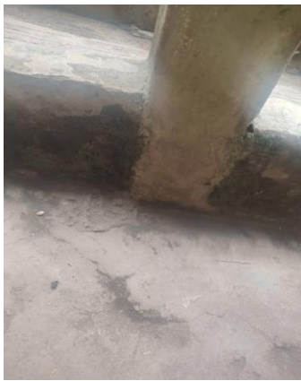
Fig. 2 Crack at the foundation
