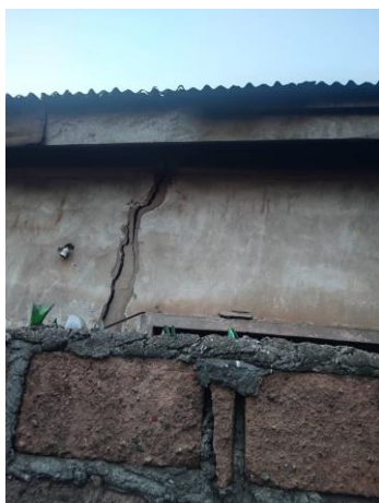
Fig.6 Crack on the wall
