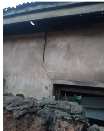
Fig.3 Crack around the beam
