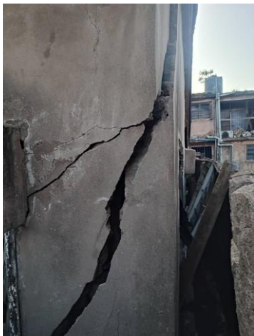
Fig. 4 Diagonal crack at the column
