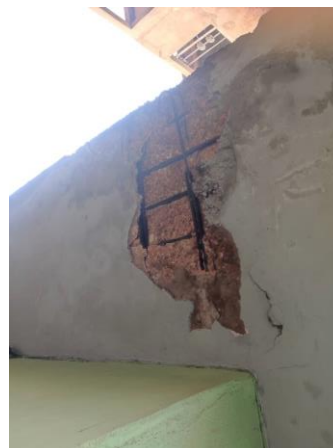
Fig.7 Crack on the decking
