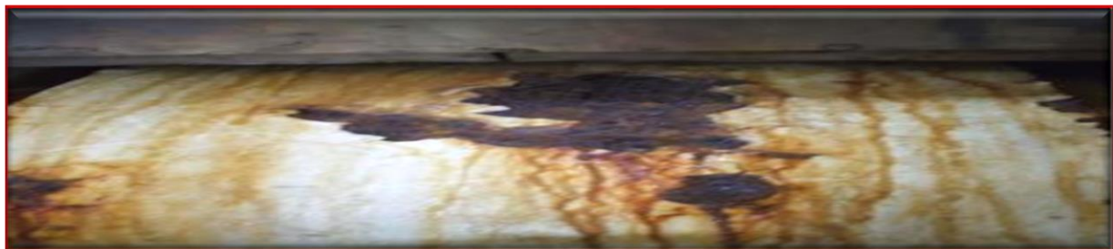
Plate I: Point on the semi-trailer shell before it was last arc-weld-repaired but later deteriorated and failed.
