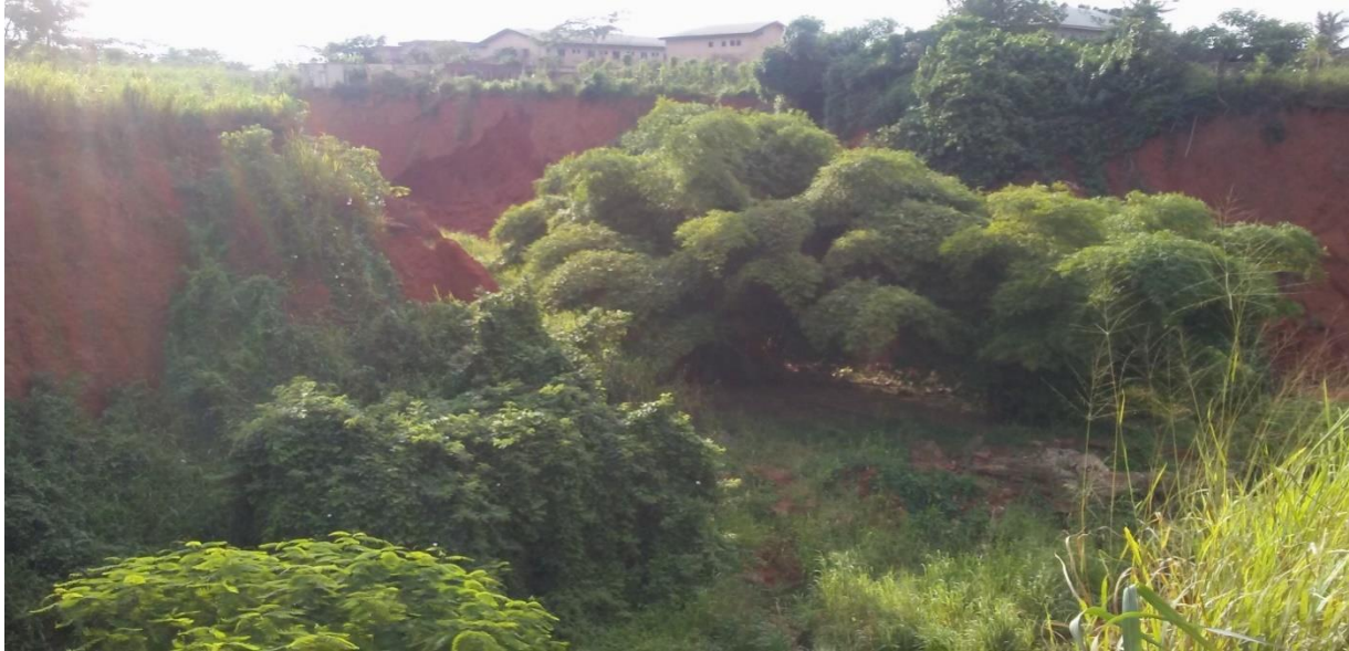
Plate 1: Gully site in University of Benin (see the buildings that are threatened)
