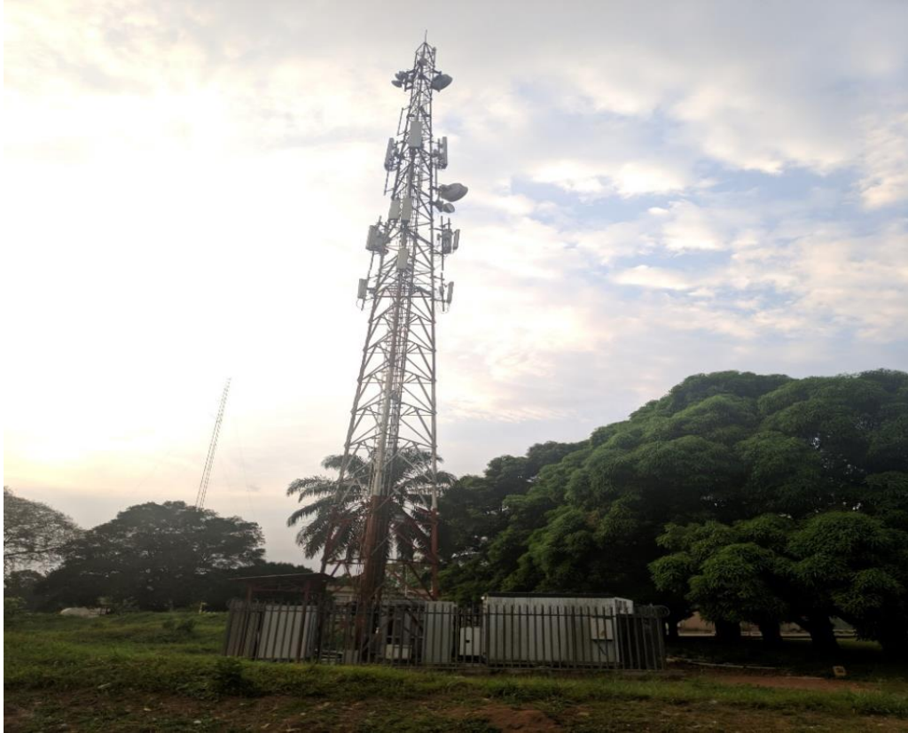
Figure 2. Physical view of the Base Transceiver Station (BTS) at engineering.
