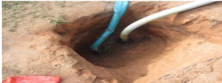
Plate 3: Carefully installed valves and hoses on Oil Export Pipeline in OML XY, by vandals
