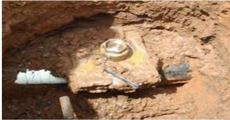
Plate 2: Carefully vandalized 6” crude oil pipeline within OML XY, by criminals
