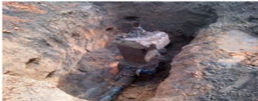
Plate 5: Valve securely mounted on crude oil export line by pipeline vandals.
