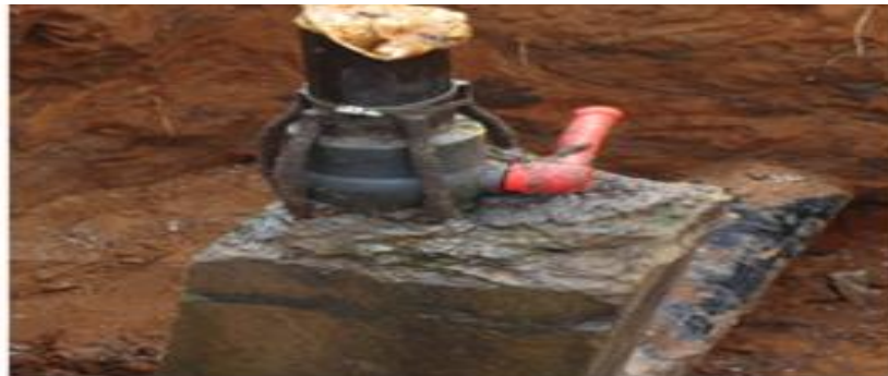
Plate 4: Concrete casting after valve installation on crude oil pipeline by pipeline vandals
