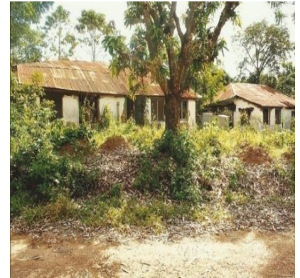
Plate 5: Houses abandoned due to cracks from seismic activity [4]
