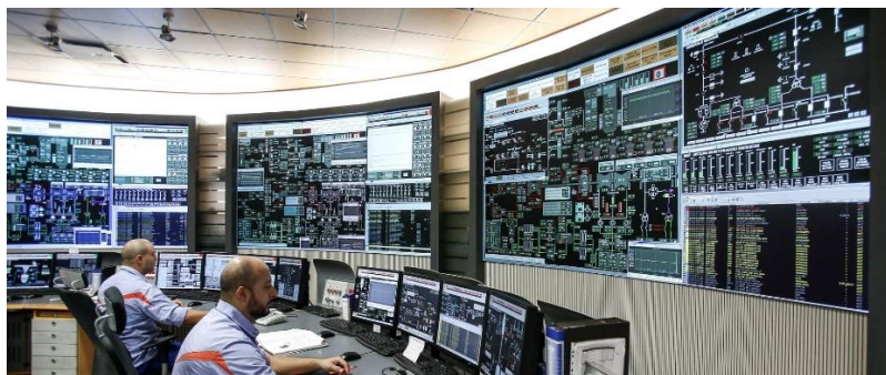
Figure 3: Control room of a power plant using SCADA
