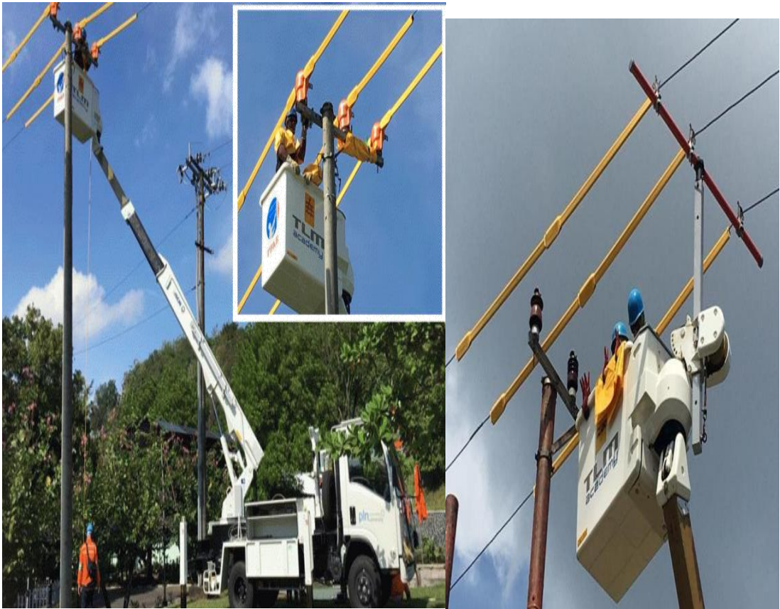
Figure 1: Installation of pedestal isolators in a stressed state Using the Direct Touch Method (source: www.pdkb.id) [10]
