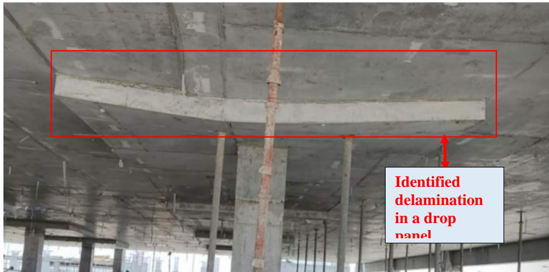
Figure 1. A visible sign of delamination of delamination
