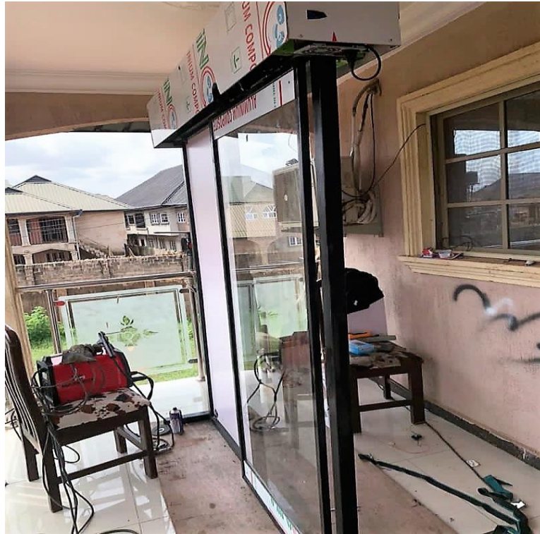
Figure 16 A pictorial view of the intelligent door with the glass sliding door
