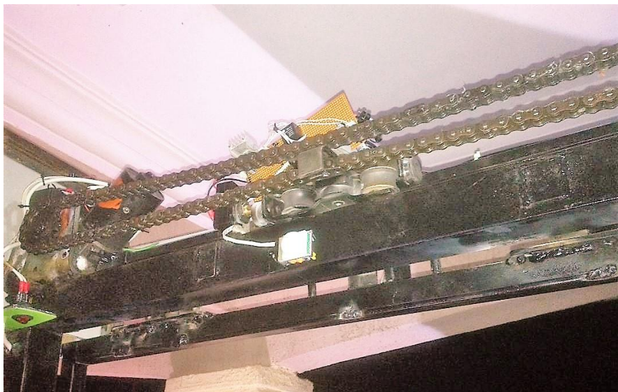
Figure 9. A pictorial view of the installed sprockets, chain, and motor
