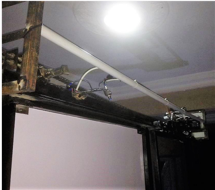
Figure 10. A pictorial view of the installed limit switches
