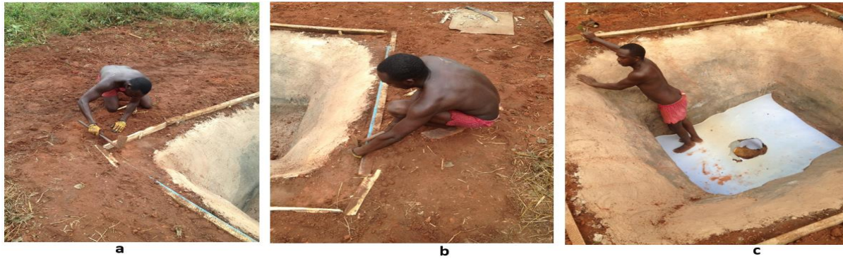
Figure 6: Preparing the interior and exterior parts of the landfill system for installation of HDPE liner
